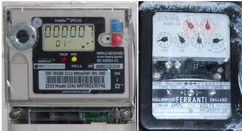
Figure 1. A typical Smart Meter and the traditional electromechanical meter it replaces
